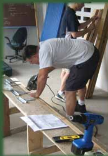
Mission team members work on the construction of the chicken coop made for the orphanage during their recent mission trip.
